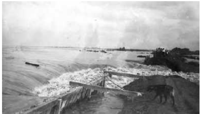
This 1891 photograph shows the work to repair the Ames Crevasse. (William S. Howell Photo Collection, Louisiana Division/City Archives, New Orleans Public Library)
